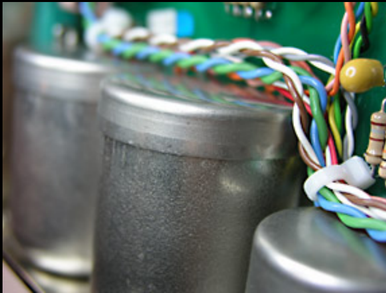
wires and transformers
